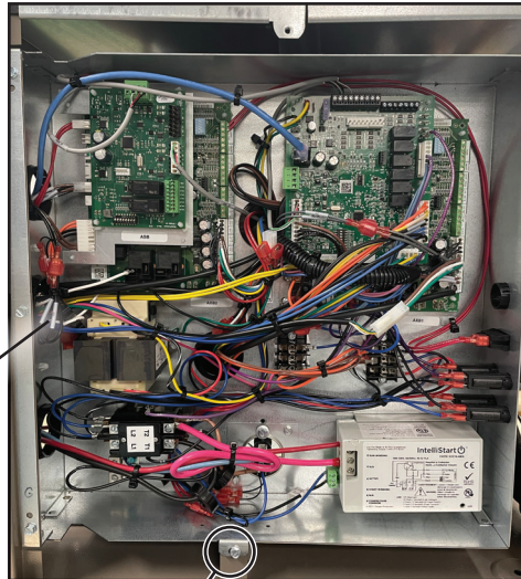
Figure 13B: Wire access (control box closed)
